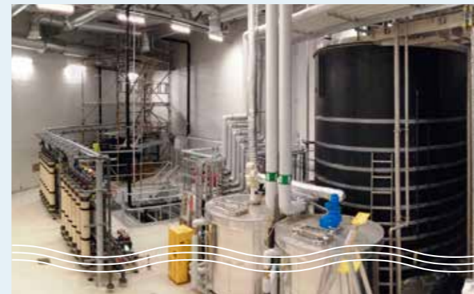
wastewater treatment plant for City of Helsingborg, RecoLab, Sweden, 2100 persons
