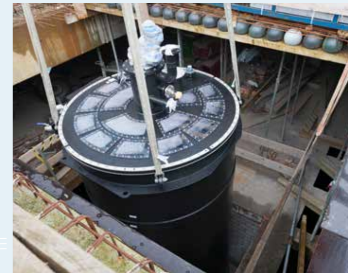
installation of black water reactor for a government office building in The Hague, NL
