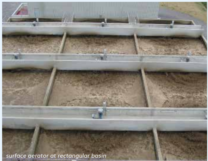
floating surface aerator
