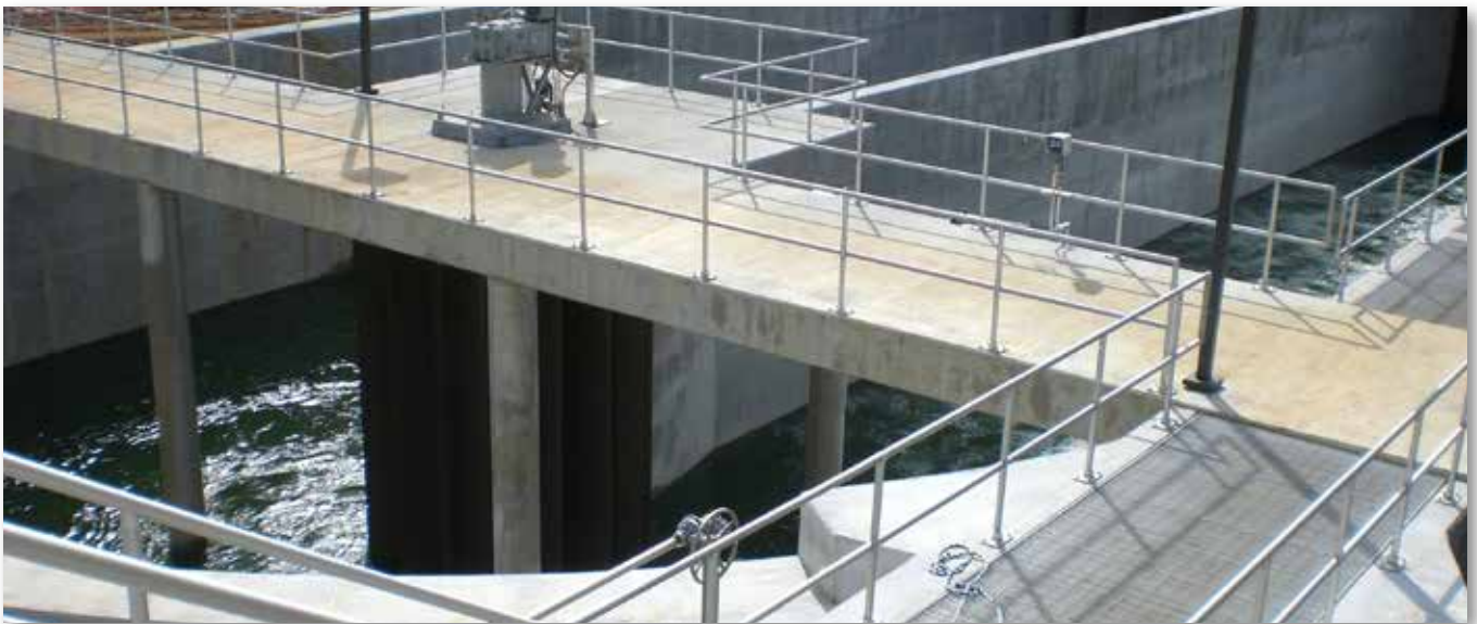
Oxidation ditch with fine bubble diffusers and Landox flow booster
