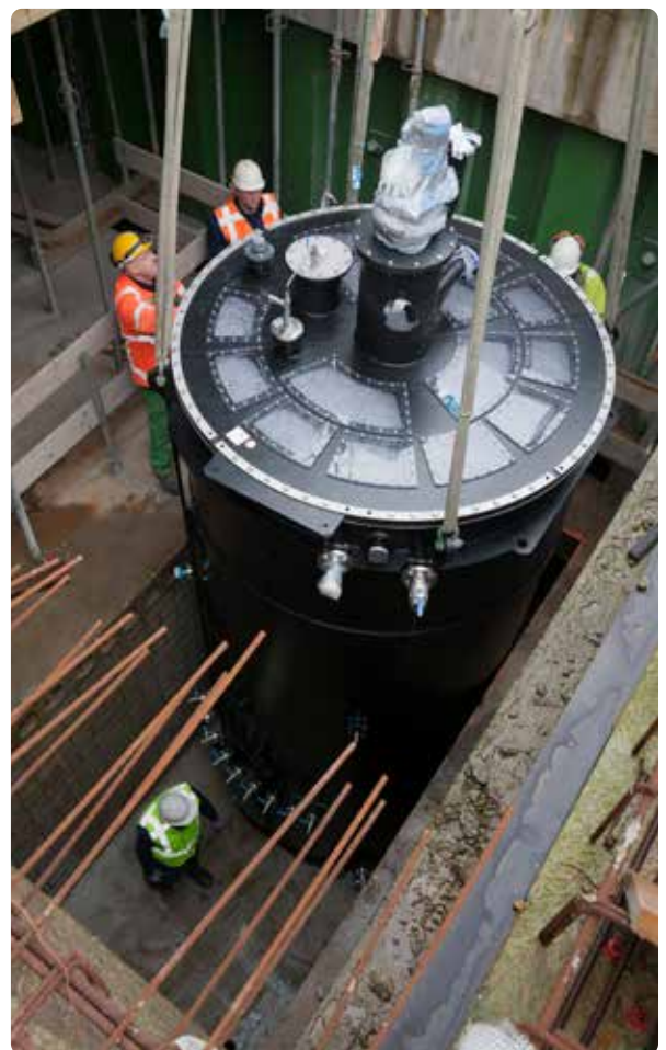
black water reactor for government office building, The Hague, NL
