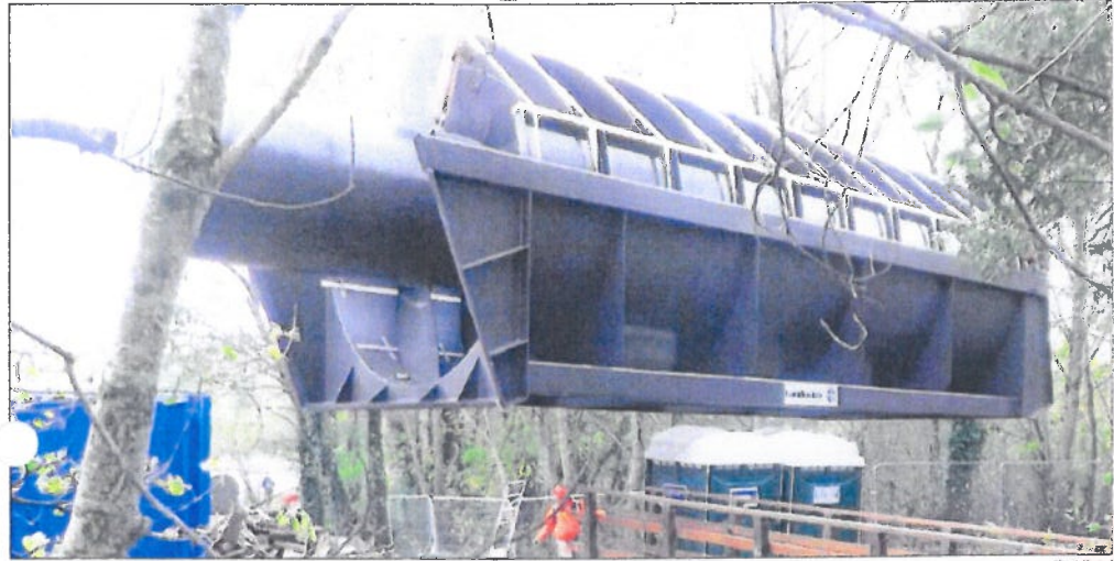
The second of two massive turbines is lifted into position at the Totnes Weir hydro-electric project. Story and more pictures on page 5
