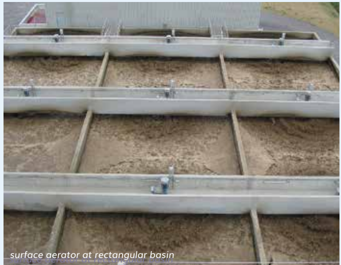
floating surface aerator
